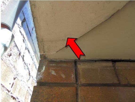
Photo 1. Exterior, female toilet, eaves – asbestos-containing fibre cement sheeting.
