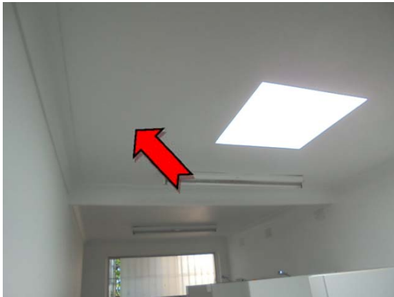
Photo 3. Interior, ground level, female toilet, ceiling – assumed asbestos-containing fibre cement sheeting.
